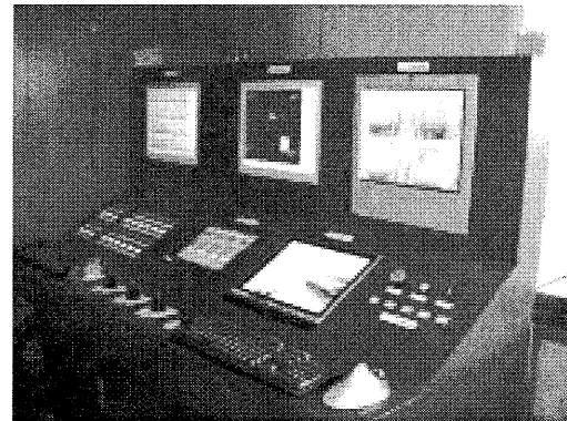
Figure 6 Remote monitoring and control panel
